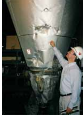
Hammer damage to hoppers impairs flow.
