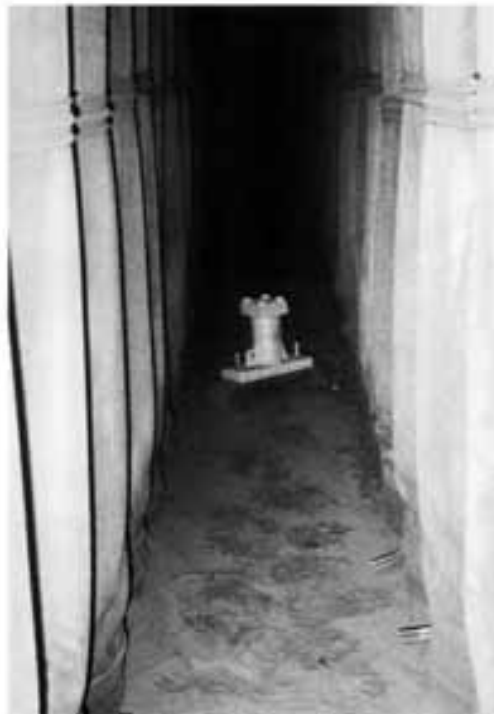
Shown here is 1 of 21 vibrators installed on the tube sheets to keep dust from building up.
