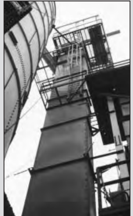
Mill Duty Bucket Elevator at a leading cement manufacturer.
